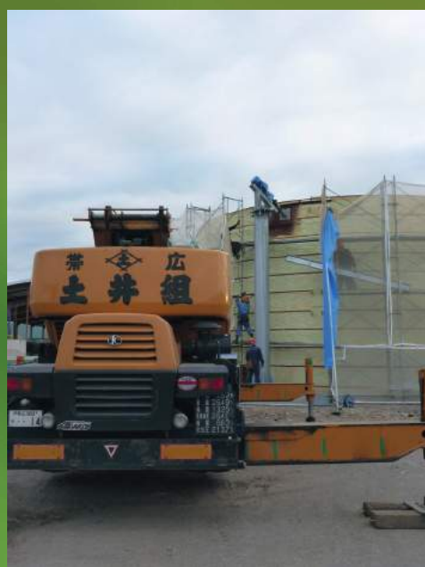
Picture: Installation of Streisal Biobull® agitator with external support column
